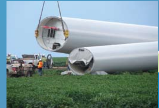
enXco contractors hoist the mid-section of a turbine tower in preparation for assembly.
